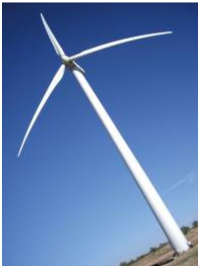
Energy production in wind power installations has many advantages.
