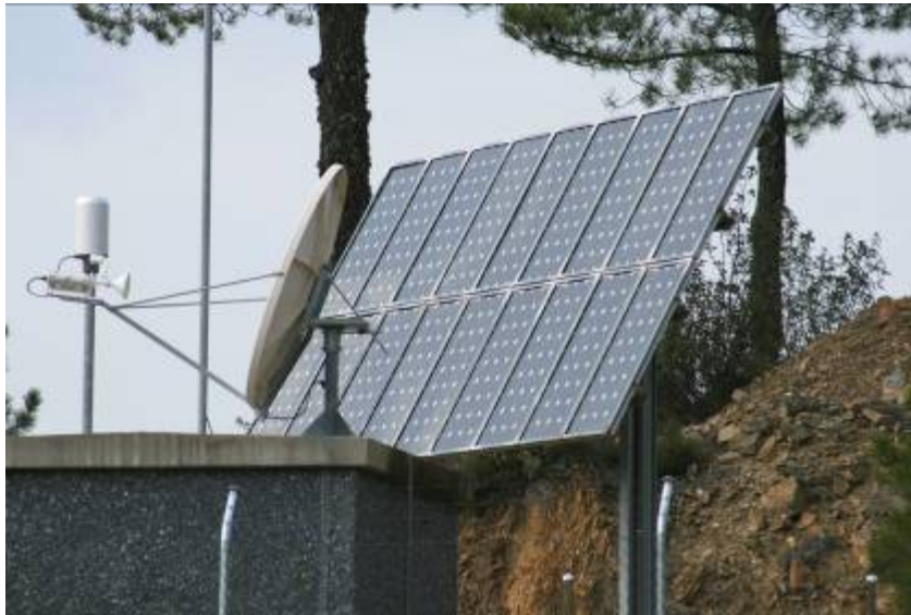
Thermal solar strings.
