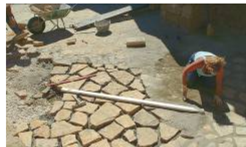
Recovery of the ruins of the Benegorri Church, built in Romanesque style.
